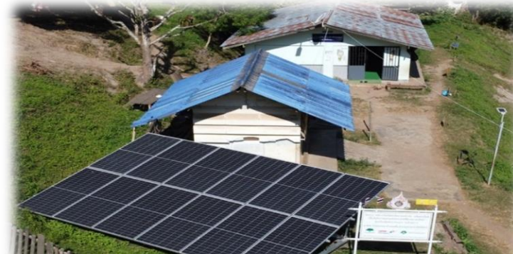
PV Off grid Project
